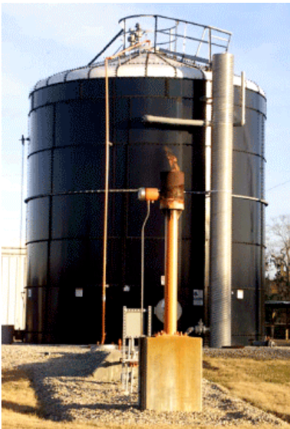
Fig. 12. Fixed-film anaerobic waste digester for methane production at the University of Florida. Photo courtesy of A. Wilkie.
